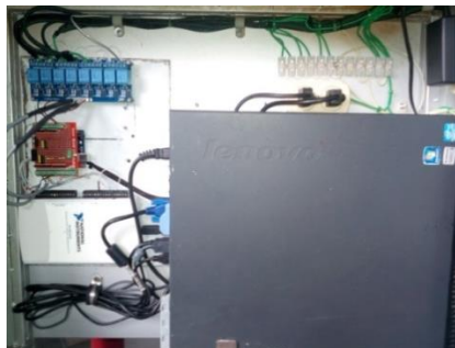
Figura 17-3: Tablero de control
