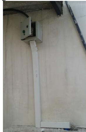
Figura 36. Control bomba cisterna 1
