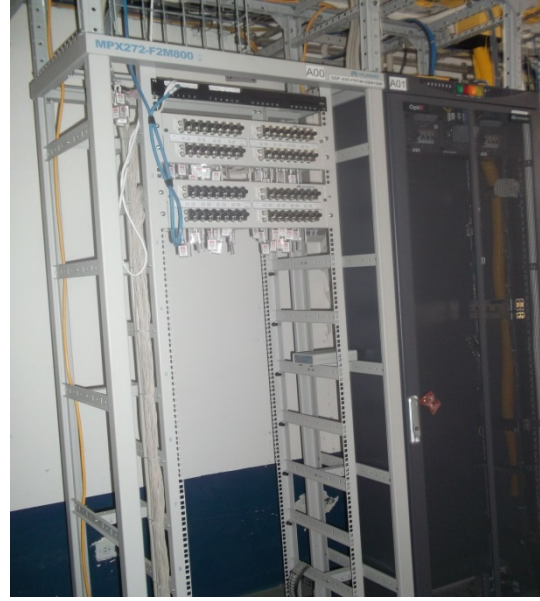
Optical Distribution Frame
