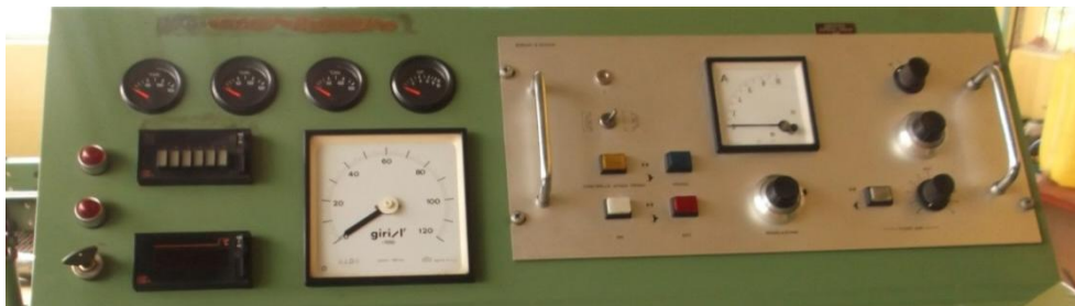
Figura 11. Panel de control
