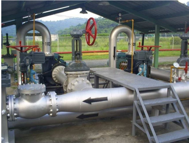
Figura 3.13: Bombas Booster P 109 110
