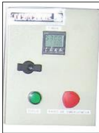
Figura 7-2: Tablero de control
