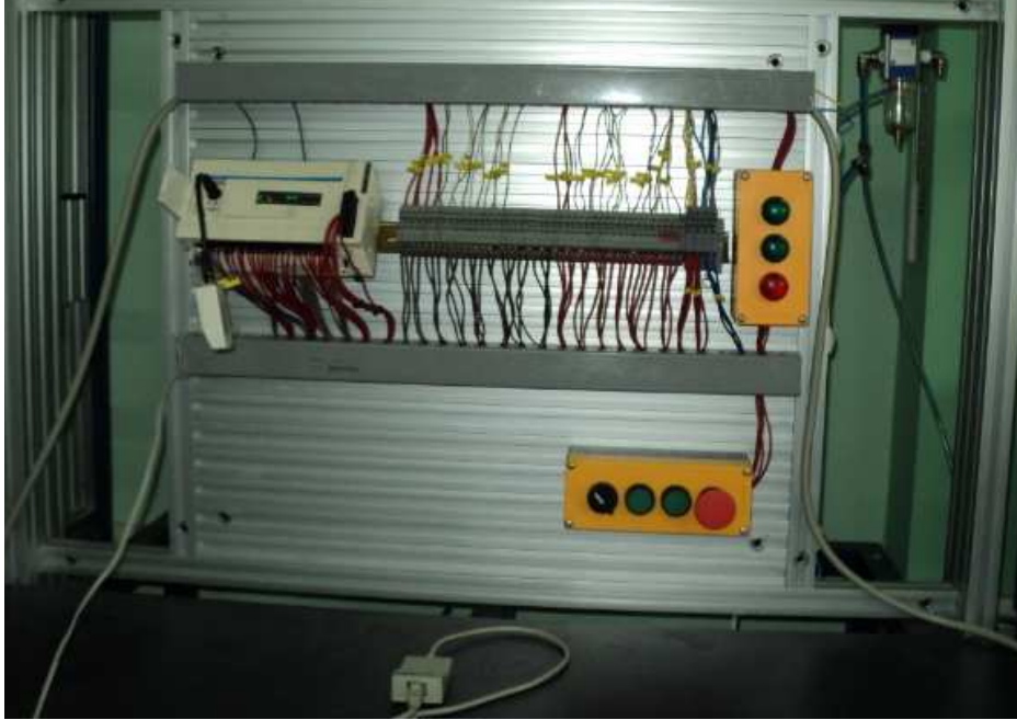
Figura 20-Cap.IV PANEL DE CONTROL
